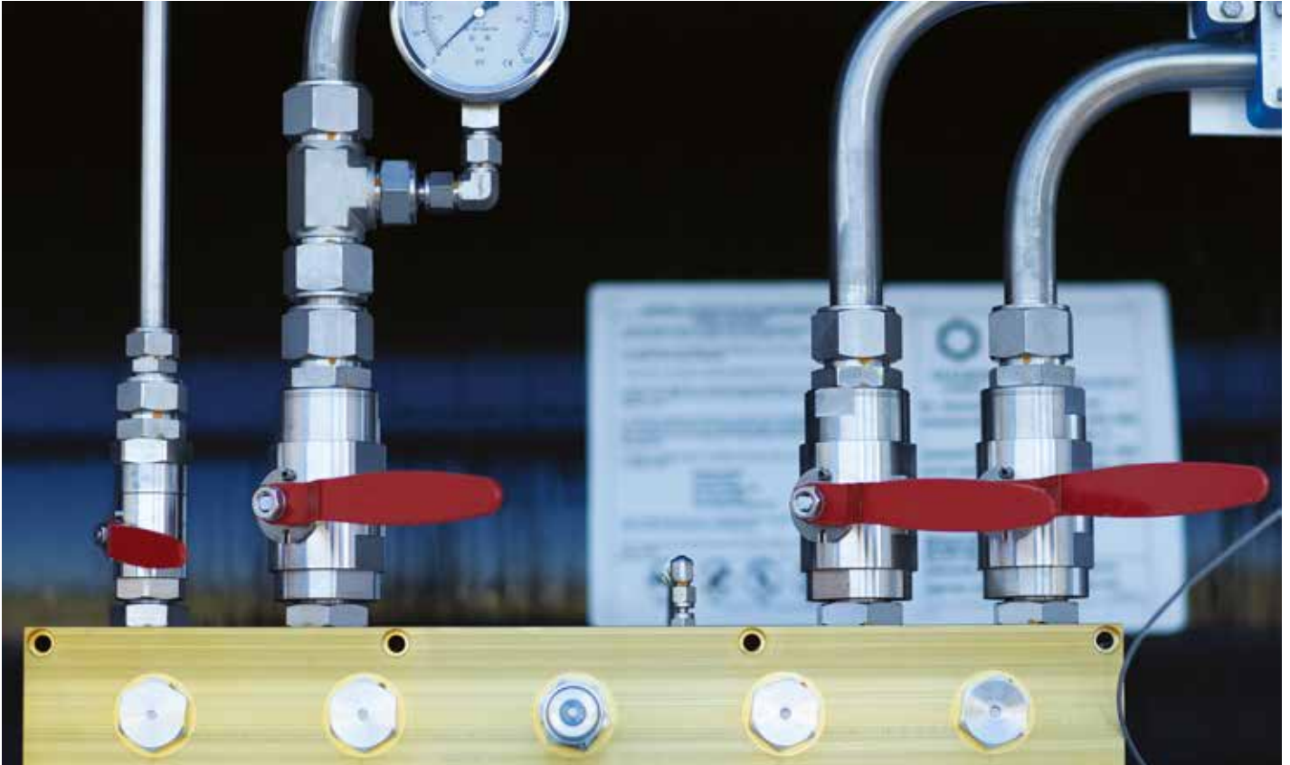
Superior plumbing delivers large quantities of gas at a high flow rate.
